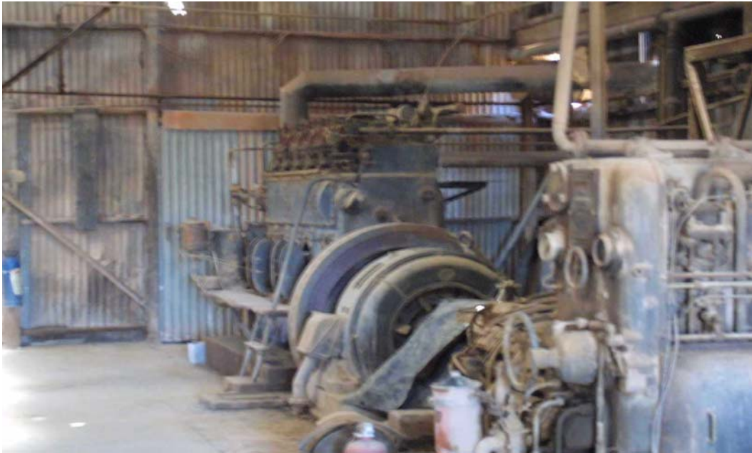
Comet Mine Power Station engines, restoration of two engines is now complete
